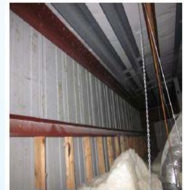
Attic Wall Lack Insulation
